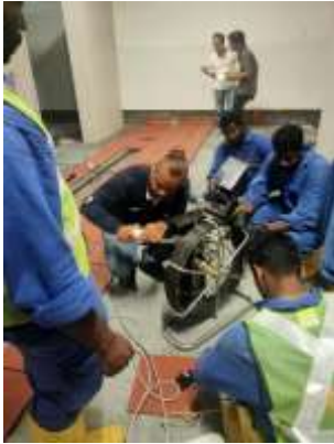
Estate executives and specialists working afterhours to localise pipe choke with specialised equipment.
