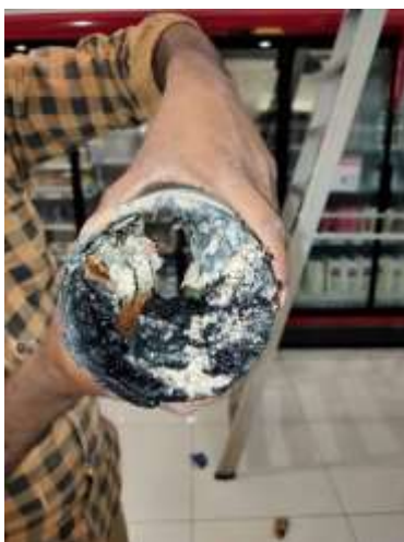
Pipe blockage localised within tenant space, within the false ceiling.
