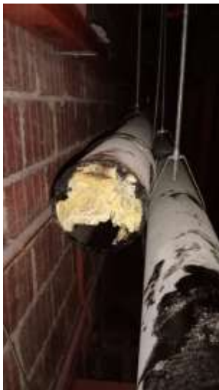
Pipe Choke discovered behind walls only accessible via tenant space.
